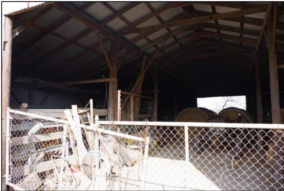
Photograph F-120: View of the interior of Resource 25a, camera facing north.
