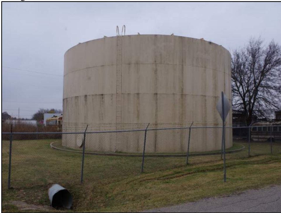
Photograph F-400: View of non-historic-age water tank associated with Resource 90, camera facing southwest.
