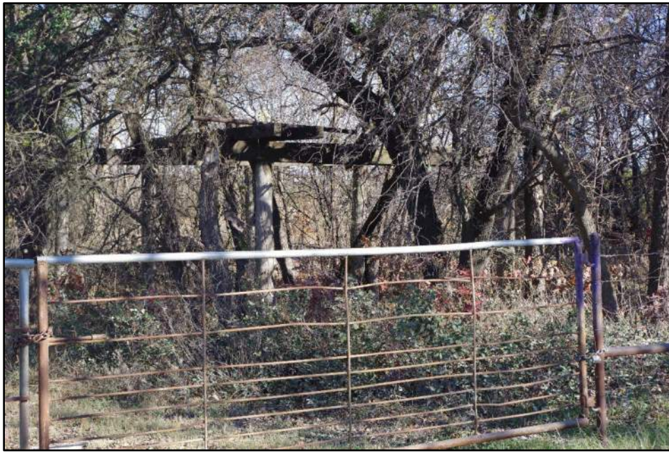
Photograph F-113: View of collapsed structure associated with Resource 23, camera facing northeast.
