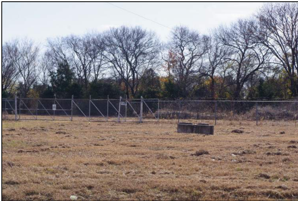
Photograph F-138: View of foundation remnant associated with Resource 29, camera facing south.
