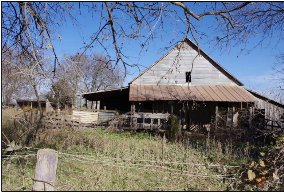
Photograph F-87: View of Resource 22b (center) and Resource 22e (left), camera facing north.
