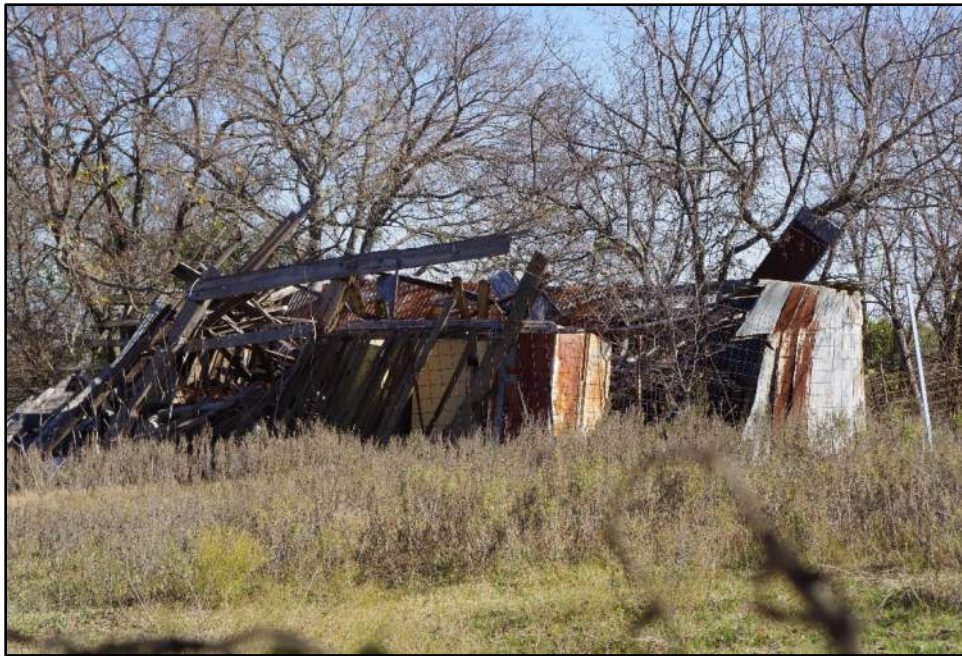
Photograph F-125: View of collapsed structure associated with Resource 25, camera facing east-northeast.
