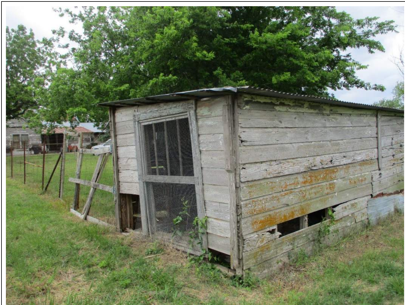
Photograph 2: View of resource 01c and 01a in to the rear, facing southwest.
