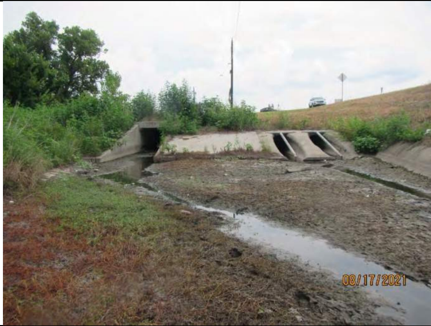
Photo 93. Photo of Emergent Wetland Water Feature 194 located in the north central portion of the Environmental Footprint. Dominant vegetation included swamp smartweed and broad-leaf cattail. Water Feature 194 is within a constructed stormwater runoff area adjacent to US 75. Photo was taken to the northeast on August 17, 2021.
