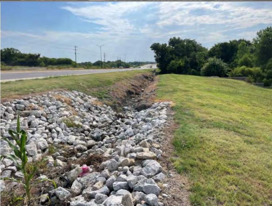
Photo 8. Photo of Ditch Drainage Feature Water Feature 10 located in the western portion of the Environmental Footprint. Water Feature 10 was constructed in uplands and drained east into Water Feature 11 . Photo was taken to the east on August 17, 2021.
