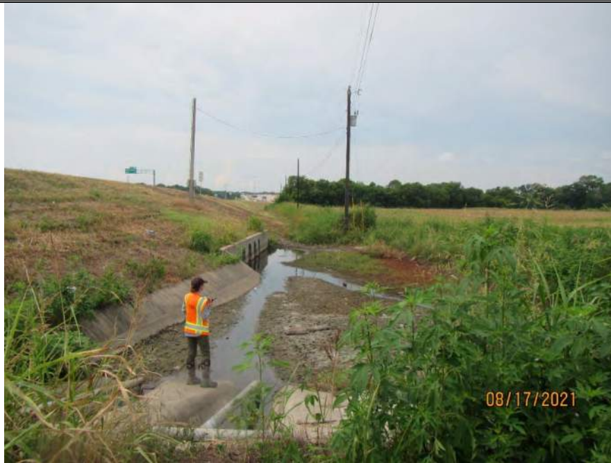
Photo 94. Photo of Swale Drainage Feature Water Feature 195 in the foreground of the photo. Ditch Drainage Feature Water Feature 193 in the background. These features were located within the central portion of the Environmental Footprint. Note how these features aided in the draining of stormwater from adjacent US 75. Photo was taken August 17, 2021.
