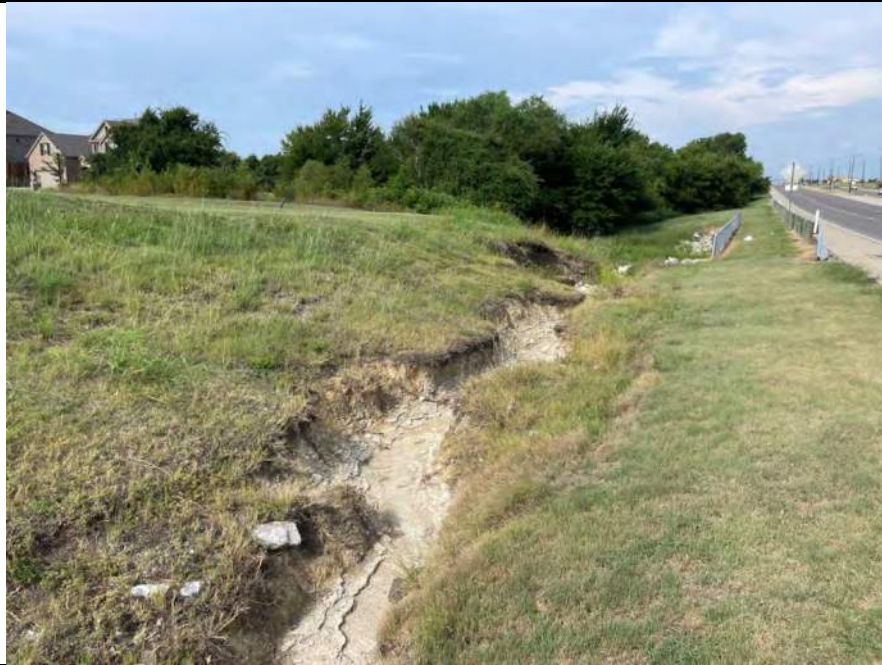
Photo 11. Photo of Ditch Drainage Feature Water Feature 22 in the western portion of the Environmental Footprint. Photo is representative of Ditch Drainage Feature Water Feature 23 . Note the erosion and adjacency to US 380. Photo was taken to the west on August 17, 2021.
