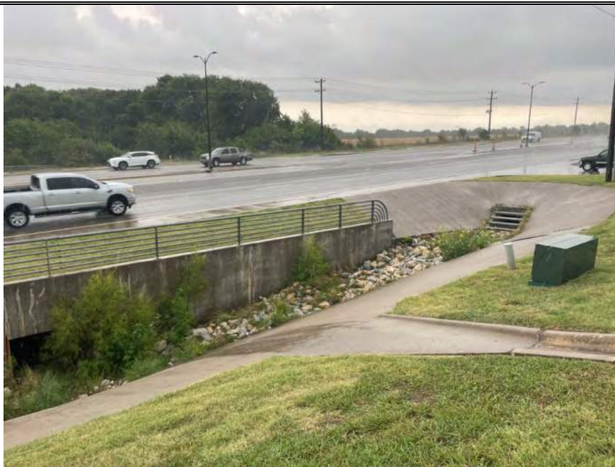
Photo 18. Photo of Ditch Drainage Feature Water Feature 35 located in the western portion of the Environmental Footprint adjacent to US 380. Water Feature 35 had riprap to control erosion. Water Feature 35 flowed north through a box culvert into Water Feature 37 . Photo taken to the northeast on August 17, 2021.
