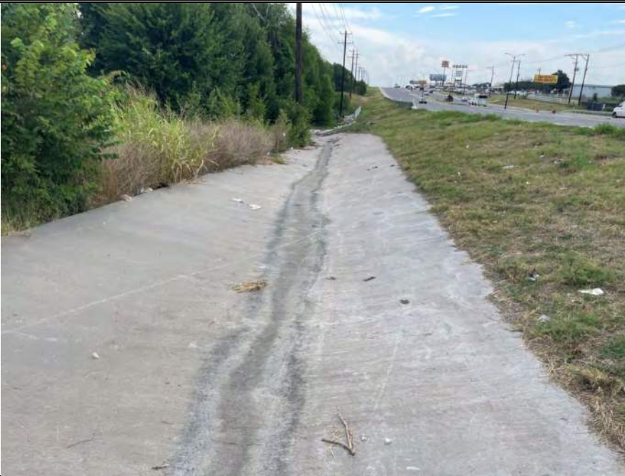
Photo 14. Photo of Ditch Drainage Feature Water Feature 29 located in the western portion of the Environmental Footprint adjacent to US 380. Water Feature 29 was lined with concrete to prevent erosion. Photo was taken to the east on August 17, 2021. Photo is representative of Ditch Drainage Features Water Feature 44, 49, and 75.
