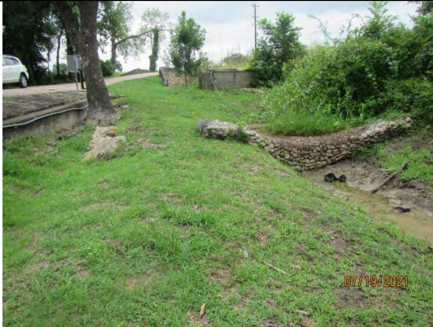
Photo 66. Photo of Ephemeral Stream Water Feature 139 located in the western portion of the Environmental Footprint. Water Feature 139 receives roadway runoff and flows northeast into Water Feature 140 . Note the erosion control structure in place and matted vegetation. Dominant riparian vegetation included bermudagrass, johnsongrass, and Chinese privet. Photo was taken to the southwest on July 19, 2021.
