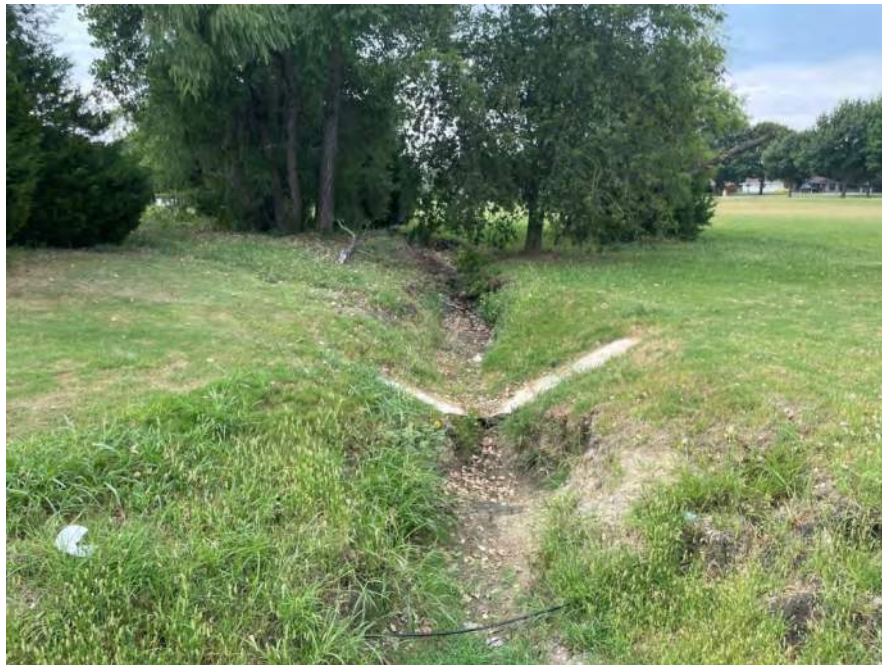
Photo 12. Photo of Ephemeral Stream Water Feature 25 located in the western portion of the Environmental Footprint. Note the lack of water within the defined channel and eroded banks. Dominant riparian vegetation was bermudagrass. Photo was taken to the south on August 17, 2021.
