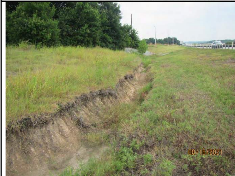
Photo 109. Photo of Ditch Drainage Feature- Water Feature 216 in the central portion of the Environmental Footprint. Water Feature 216 was constructed in uplands to aid in the removal of stormwater runoff from US 75. Note the presence of erosion here. Photo was taken to the west on August 16, 2021.
