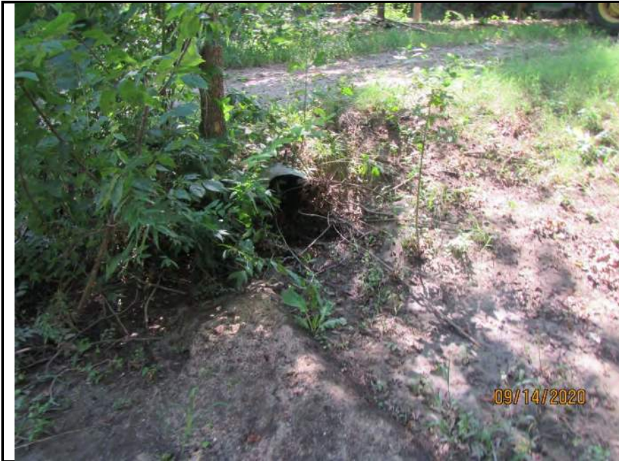
Photo 144. Photo of Swale Drainage Feature Water Feature 328 in the eastern portion of the Environmental Footprint. Note the lack of an OHWM, hydrophytic vegetation, hydric soils, hydrological indicators, a stream bed, or banks. Photo was taken September 14, 2020.
