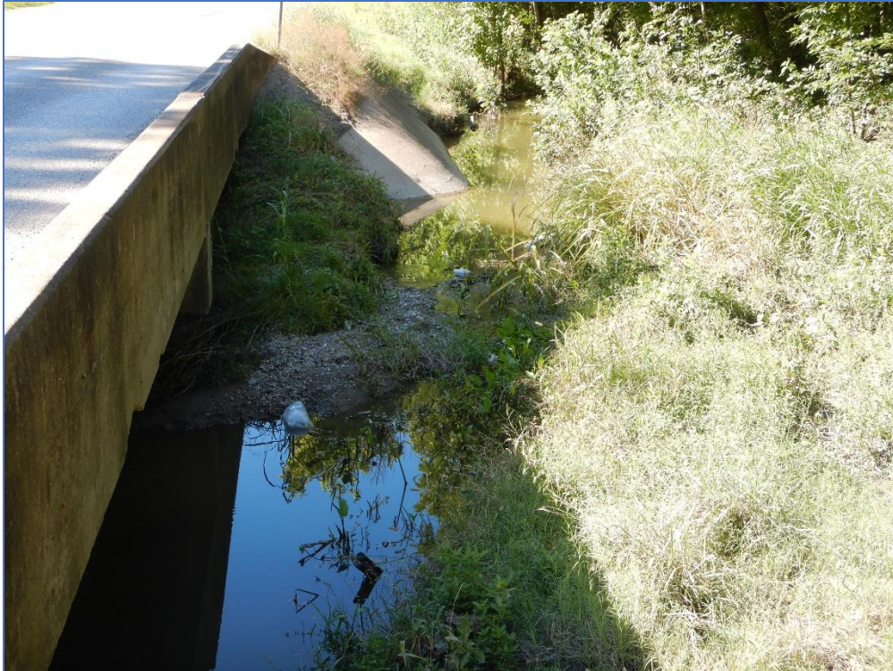
Photo 33. Drainage by Griffin Lane on the east side of FM 741; view north.
