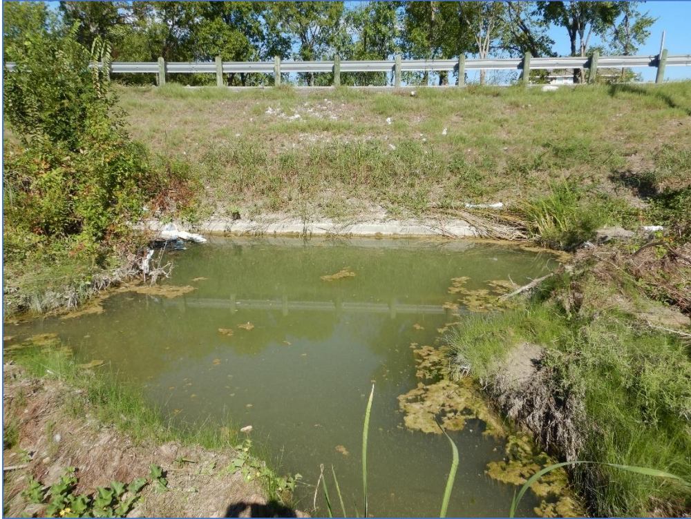
Photo 31. Channelized drainage on east side of FM 741 by Bronte Blvd; view northwest.
