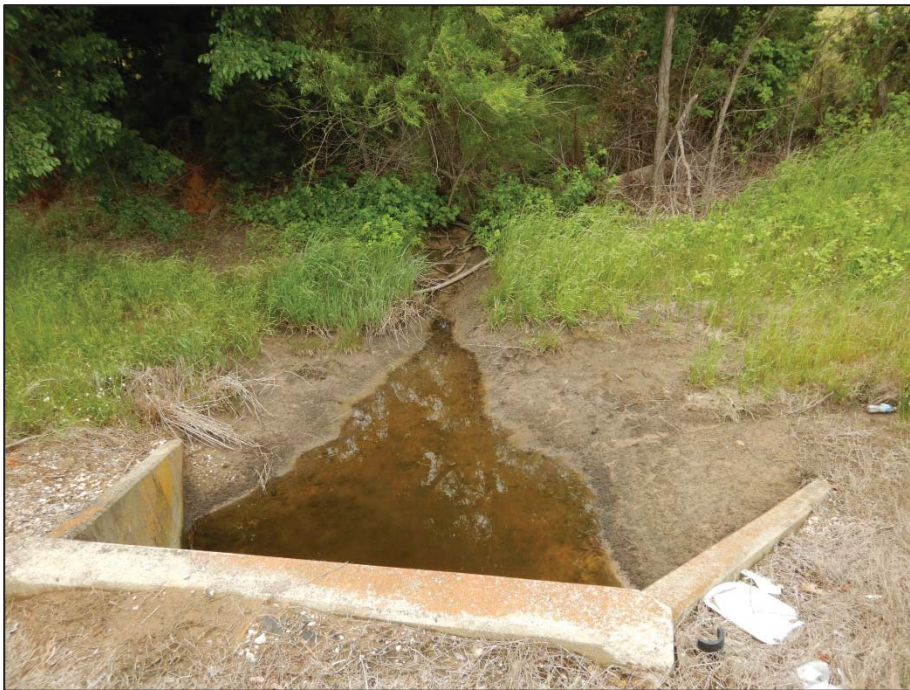
Photo 82: View looking northwest toward Crossing 11 – tributary to Pecan Creek (US 377 southbound side).
