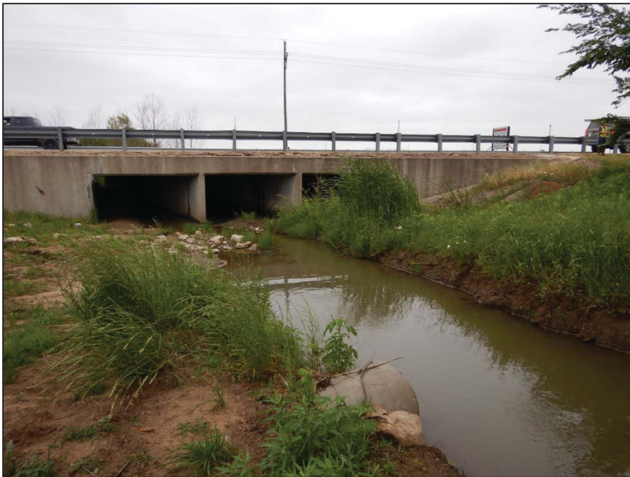
Photo 54: View looking east toward Crossing 3 – tributary to Pecan Creek (US 377 southbound side).
