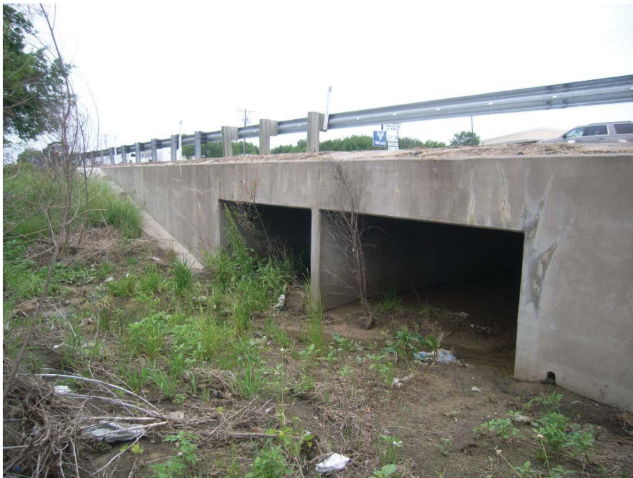
Photo 50: View looking west toward Crossing 2 – tributary to Pecan Creek (US 377 northbound side).
