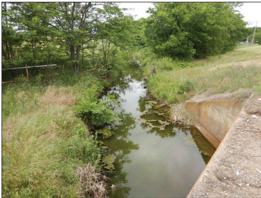
Photo 94: View looking northwest toward Crossing 14 – tributary to Pecan Creek (US 377 southbound side).
