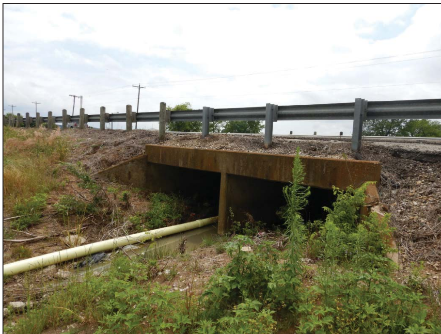
Photo 101: View looking west toward Crossing 16 – tributary to Cantrell Slough (US 377 northbound side).
