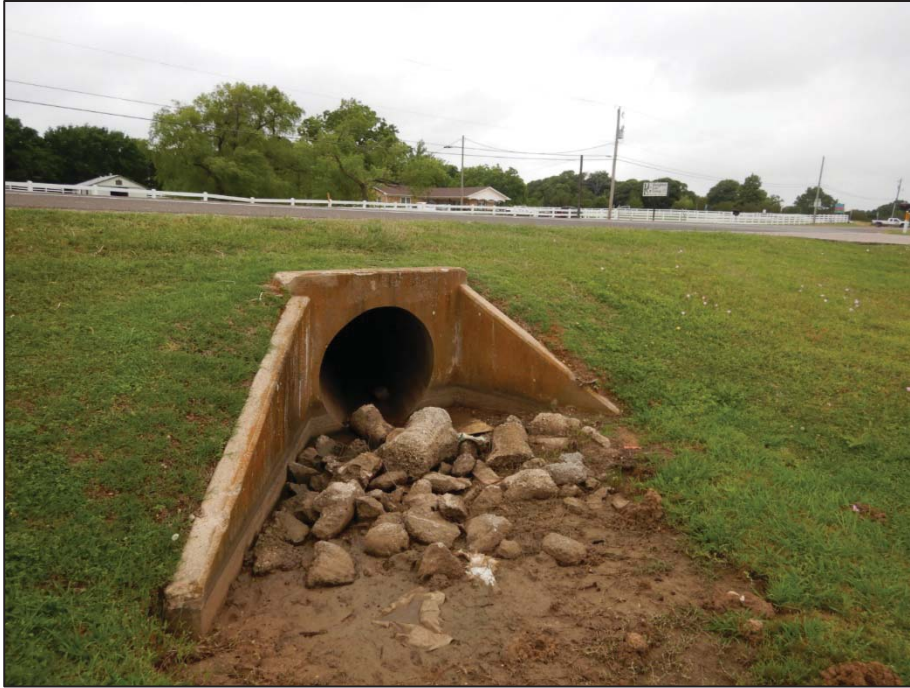
Photo 75: View looking northwest toward Crossing 9 – tributary to Pecan Creek (US 377 southbound side).
