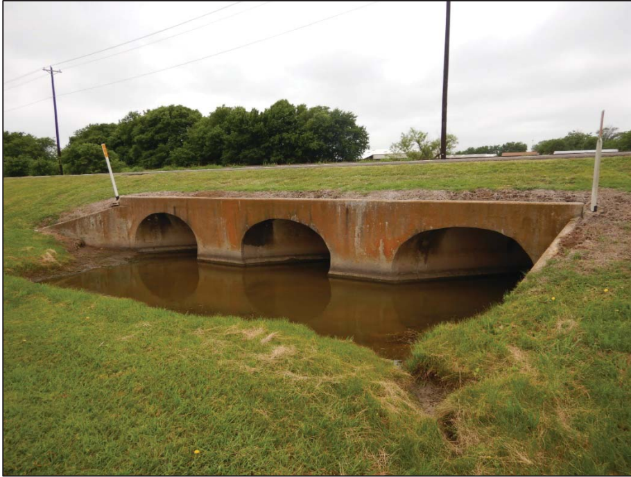
Photo 73: View looking west toward Crossing 8 – tributary to Pecan Creek (US 377 northbound side).
