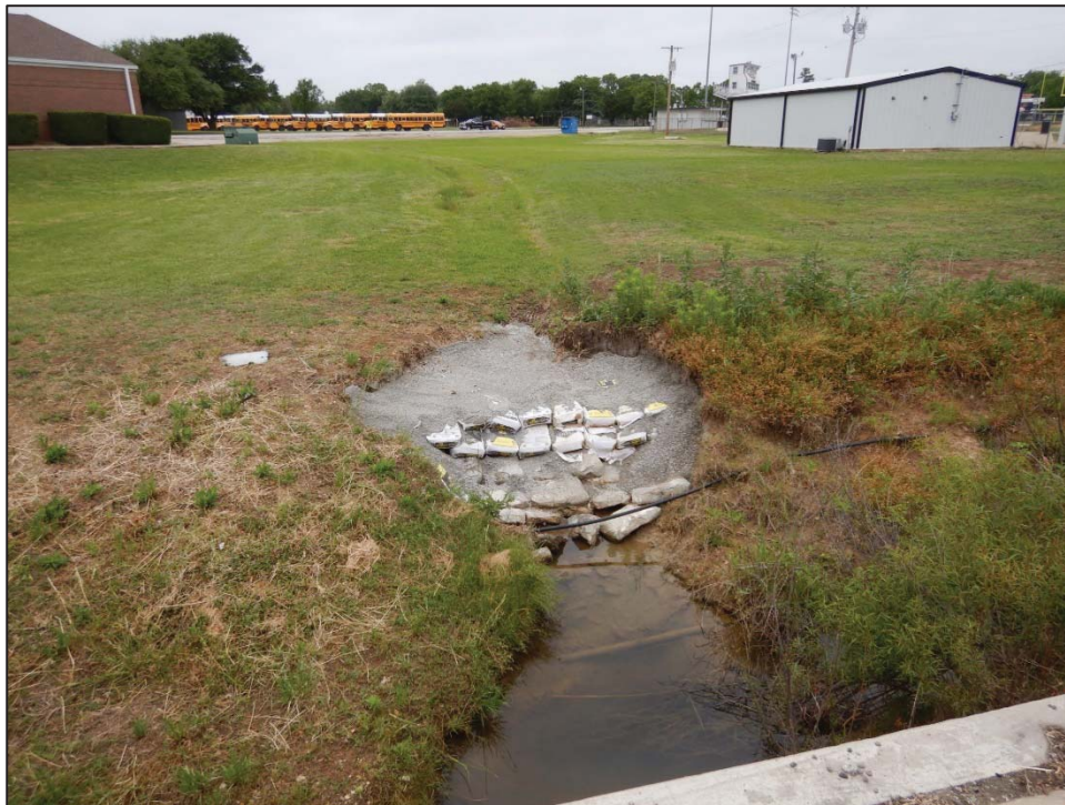
Photo 58: View looking northwest toward Crossing 4 – tributary to Pecan Creek (US 377 southbound side).
