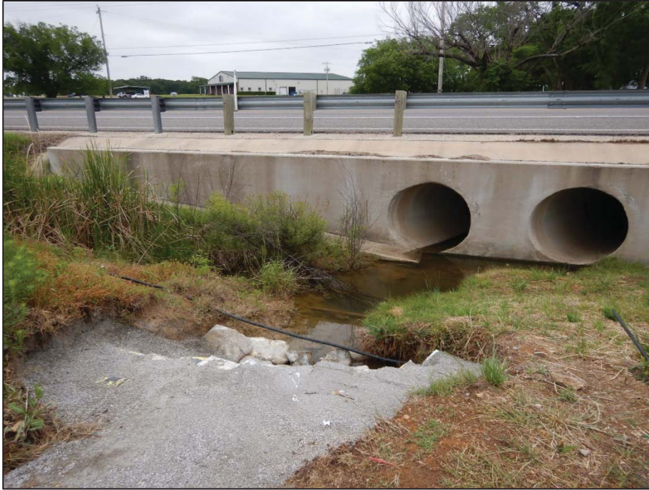
Photo 57: View looking southeast toward Crossing 4 – tributary to Pecan Creek (US 377 southbound side).
