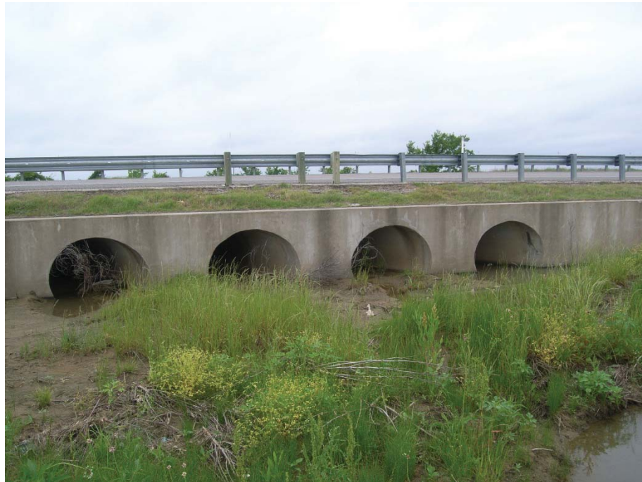
Photo 48: View looking west toward Crossing 1 – tributary to Pecan Creek (US 377 northbound side).
