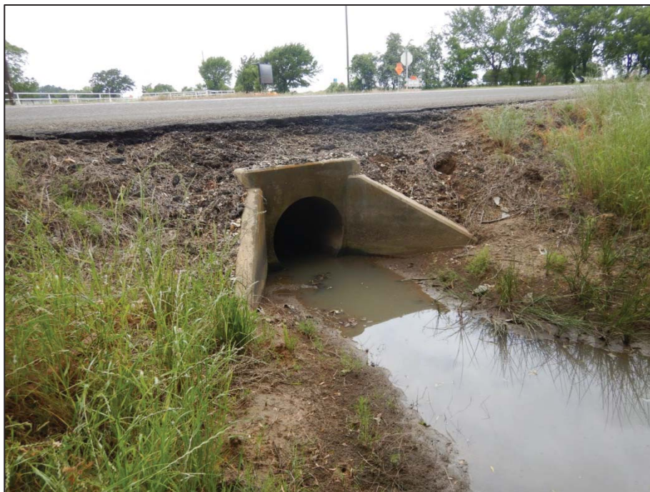
Photo 97: View looking west toward Crossing 15 – tributary to Cantrell Slough (US 377 northbound side).
