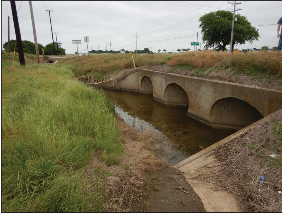
Photo 71: View looking east toward Crossing 8 – tributary to Pecan Creek (US 377 southbound side).
