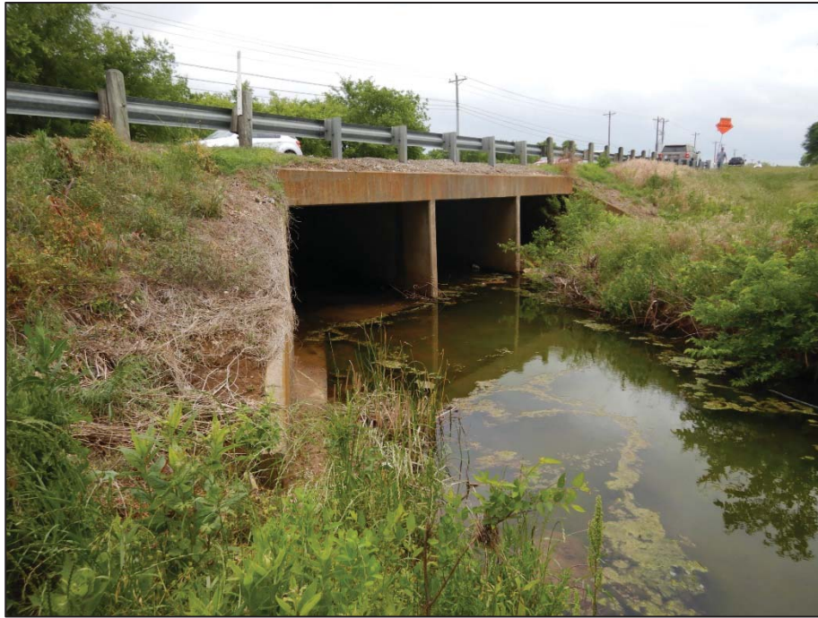
Photo 93: View looking southeast toward Crossing 14 – tributary to Pecan Creek (US 377 southbound side).
