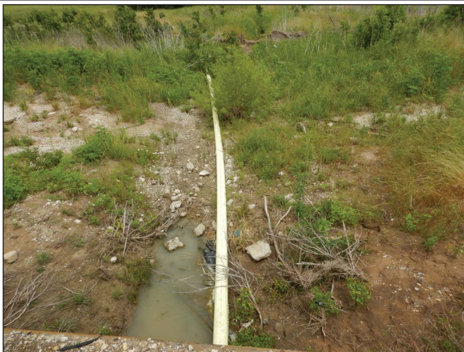
Photo 102: View looking east toward Crossing 16 – tributary to Cantrell Slough (US 377 northbound side).
