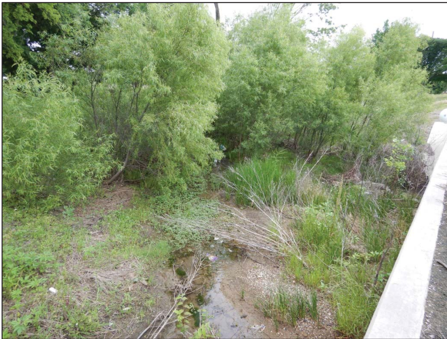
Photo 60: View looking south toward Crossing 4 – tributary to Pecan Creek (US 377 northbound side).
