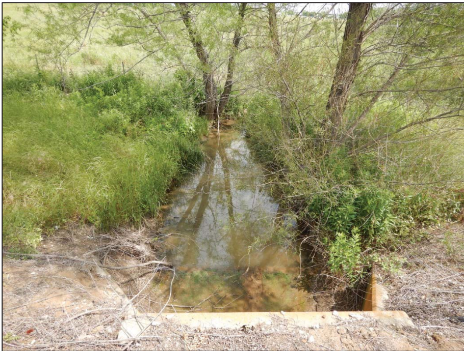
Photo 104: View looking southeast toward Crossing 17 – tributary to Cantrell Slough (US 377 northbound side).
