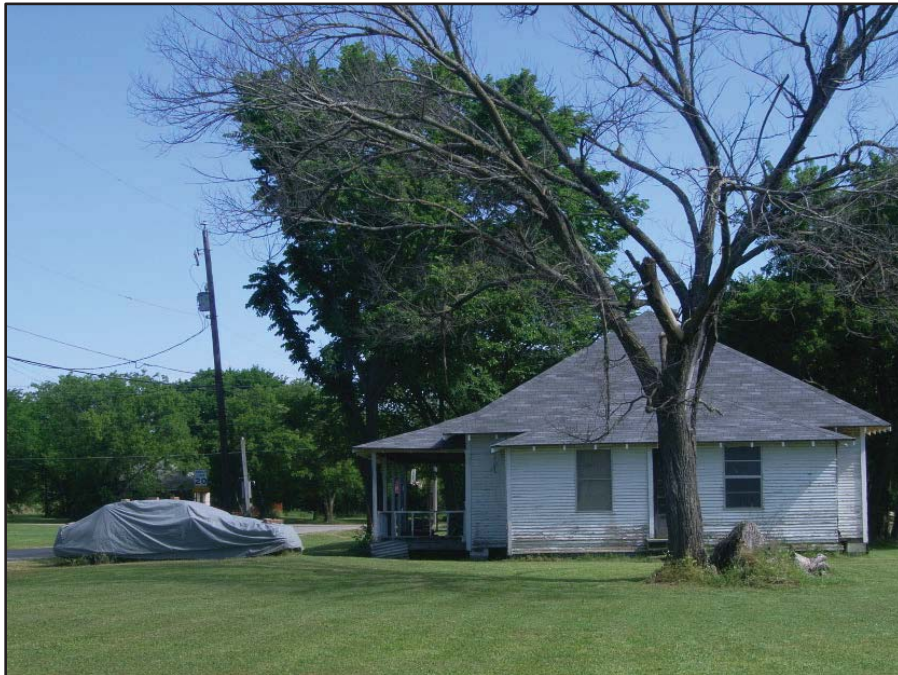
Photo 30: View looking north from E Walcott St in Pilot Point toward a home in disrepair. Date of Photo: 5/6/20
