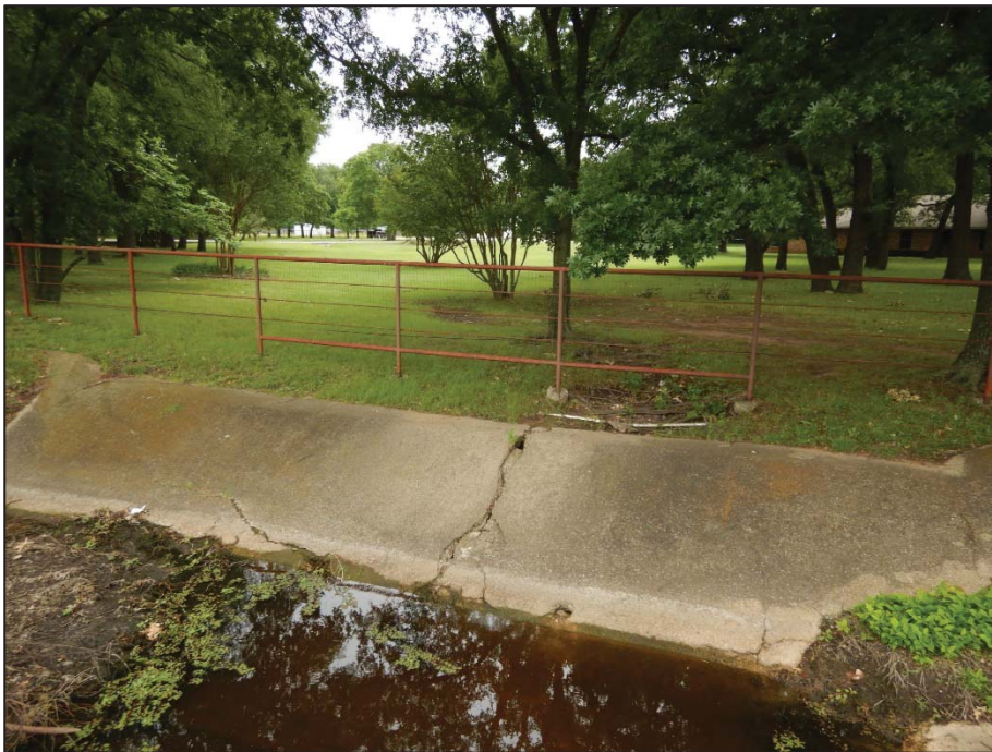
Photo 78: View looking southwest toward Crossing 10 – tributary to Pecan Creek (US 377 southbound side).
